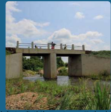
A climate-resilient bridge connects communities through the LoCAL programme. ©UNCDF/ Chrismel Wasswa
