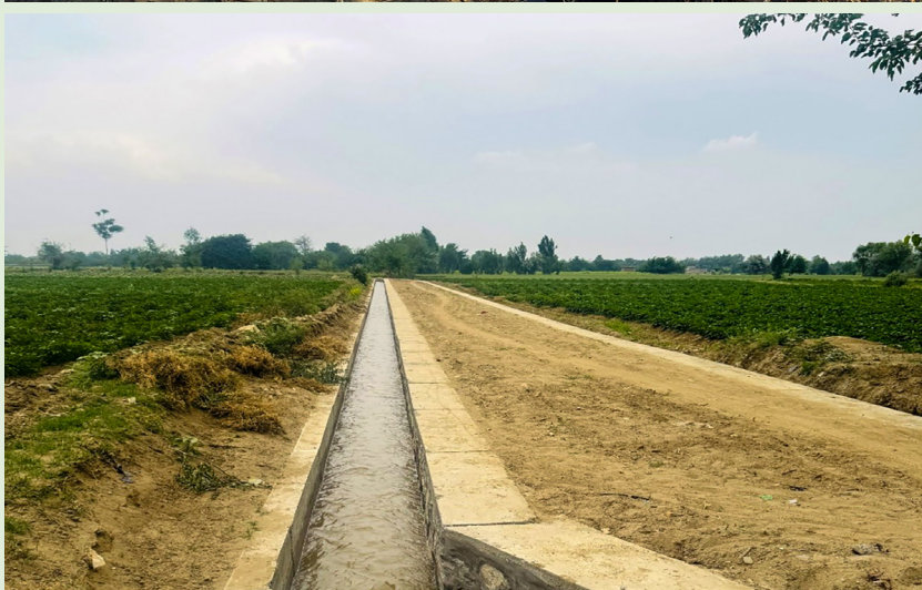
The photos show rehabilitation of Bayezed canal before (top) and after (bottom). © FAO Afghanistan
